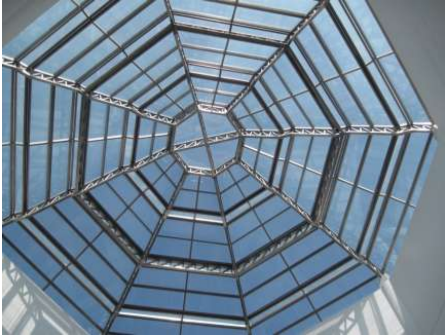
1 The Ceiling of the ceremonial hall is covered by a skylight made of glass and stainless steel
